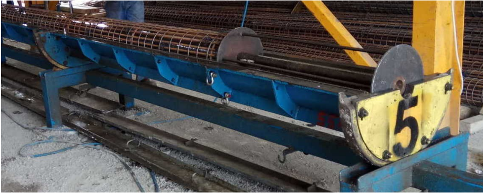
Pic. 1 Reinforcement cage within the lower half of mold ready for concreting. At the bottom of the mold the spacer to reduce the length of the pole.
